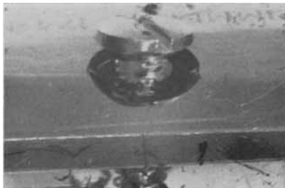
Fig. 33 b. This screw head ( \times 5 ) was deformed by the screw driver but shows hardly any corrosion. The screw hole, however, shows corrosion. The colours seen to ooze from underneath the plate around the screw come from the screw hole. This may be an example of crevice corrosion. In one of the larger areas damaged on the edge of the plate some corrosion is seen. No corrosion is seen in the stamped letters and figures.
